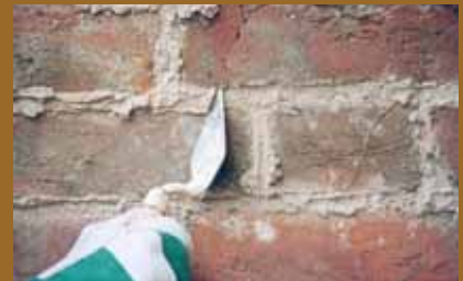
Finishing the joints first requires trimming off the surplus mortar with a small trowel or key. If the mortar is the right consistency, stains are not left on the masonry.
