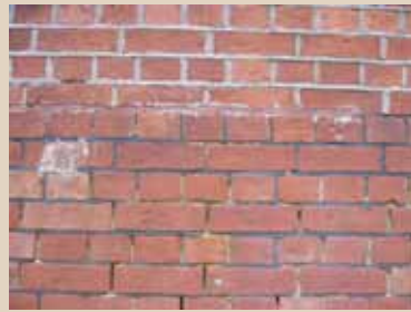
Some building types for instance those typical of military installations have distinctive mortar traditions, such as the neat black ash pointing seen in the lower courses of brick. Unfortunately the poor quality, weather-struck seen in the top courses of brick is endemic, disfiguring and damaging to the wall and distorting the evidence of the original appearance.
