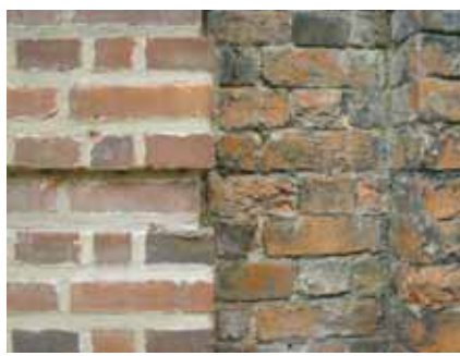
Illustrates the disastrous visual impact of replacement bricks and full, wide joints against the fine jointed early 18th Century brickwork against which it has been juxtaposed.
