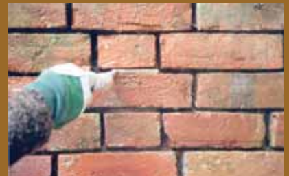
Cranked pointing keys of various widths to fit a wide variety of joints sizes are needed to point successfully. Note that the blade of the key fits easily into the joint.
