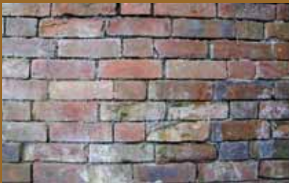
Brick panel in need of repointing.
