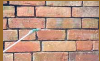
Prepared wall being washed out to remove soil, dust and debris. A back pack pressure spray fitted with a lance and adjustable nozzle is ideal. The wall must be damp until the mortar is placed.
