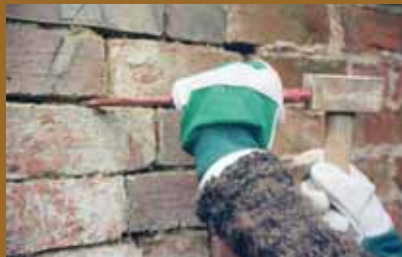
Cutting out pointing with much deteriorated mortar really only requires raking and washing out, with localised cutting out of hard spots or cement patching. When using a plugging chisel ensure the blade fits comfortably into the joint width and that cutting out is always towards a void to prevent wedging and spalling arrises.
