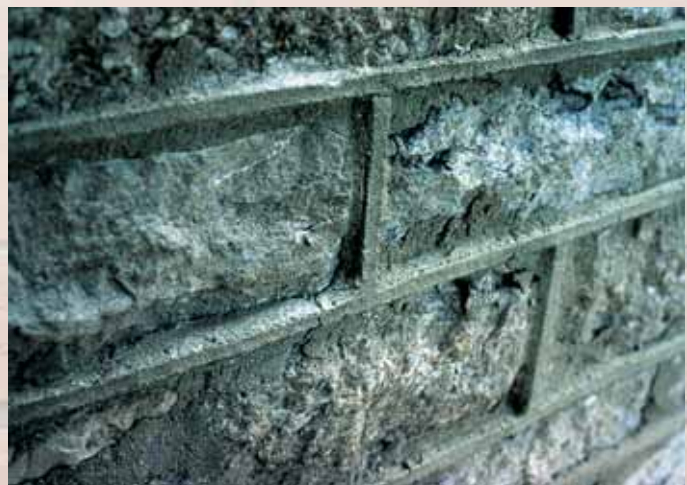
Fine jointed ashlar has been too difficult to point properly and cementitious mortar straps have been applied over the original joints, disfiguring the wall and preventing it from drying out. This is a straightforward lack of understanding and skill.
