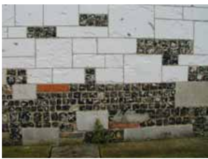
Shows chalk ashlar range work mixed with squared, knapped black flints and tiles in a cement:lime:sand composition mortar which is beginning to create problems for the permeable stone.
