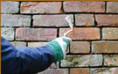
The mortar is easily picked up on the key and properly compacted. The mortar should be stiff but workable and just wet enough to stick to the blade of the pointing key and mortar board. Excessive water content is a common problem and must be avoided.
