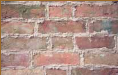
Mortar compacted into clean, damp joints. The rough appearance of the work is typical of well packed joints with mortar hanging along the arris lines. The work cannot be finished for another 12 hours and needs to be protected with plastic sheet against rapid drying.
