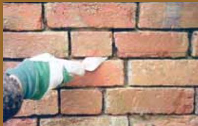
Small pointing trowels are also too wide to properly compact mortar into the joint, so that voids are often left. Trowels often leave a struck face which is inappropriate for historic work.
