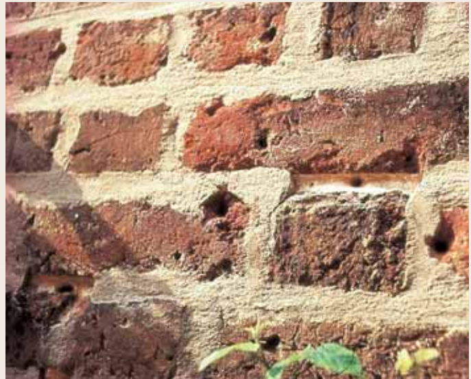
Thick, crude lime pointing plastered over original, largely sound 17th Century Brick joints. The whole appearance of the wall has been degraded unnecessarily: the original mortar, seen centre of picture, is in perfectly sound condition
