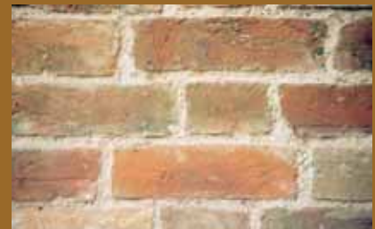
The finished panel has pointing that is simply flush but just recessed from the edges of the brick faces, with good texture, colour matching, no brush strokes.
