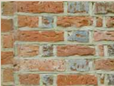
The brickwork has been hacked to receive a plaster and misaligned joints indicate filled window and door openings.
