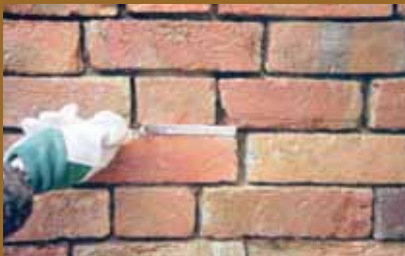
Standard brick jointers are too wide to fit into many joints with the result that mortar cannot be packed from the back of the joint. The concave profile left by this tool is often inappropriate.
