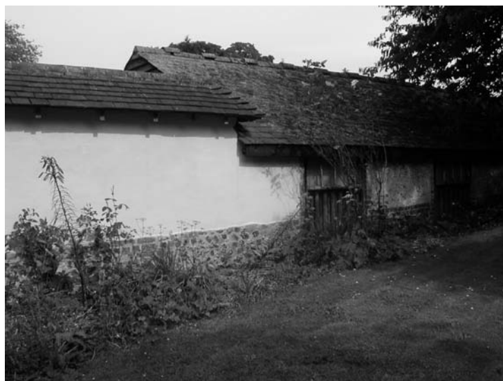
Former BaR cob wall re-built in traditional materials by National Trust, Mottisfont, Test Valley.
