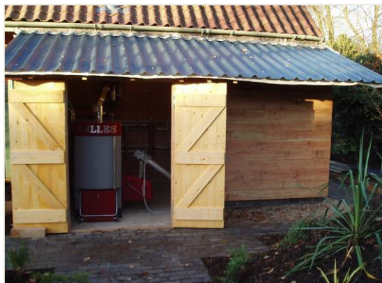
Boiler Room and Fuel Store
