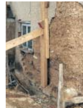
The use of hard cement render on a cob building leading to major structural failure.
