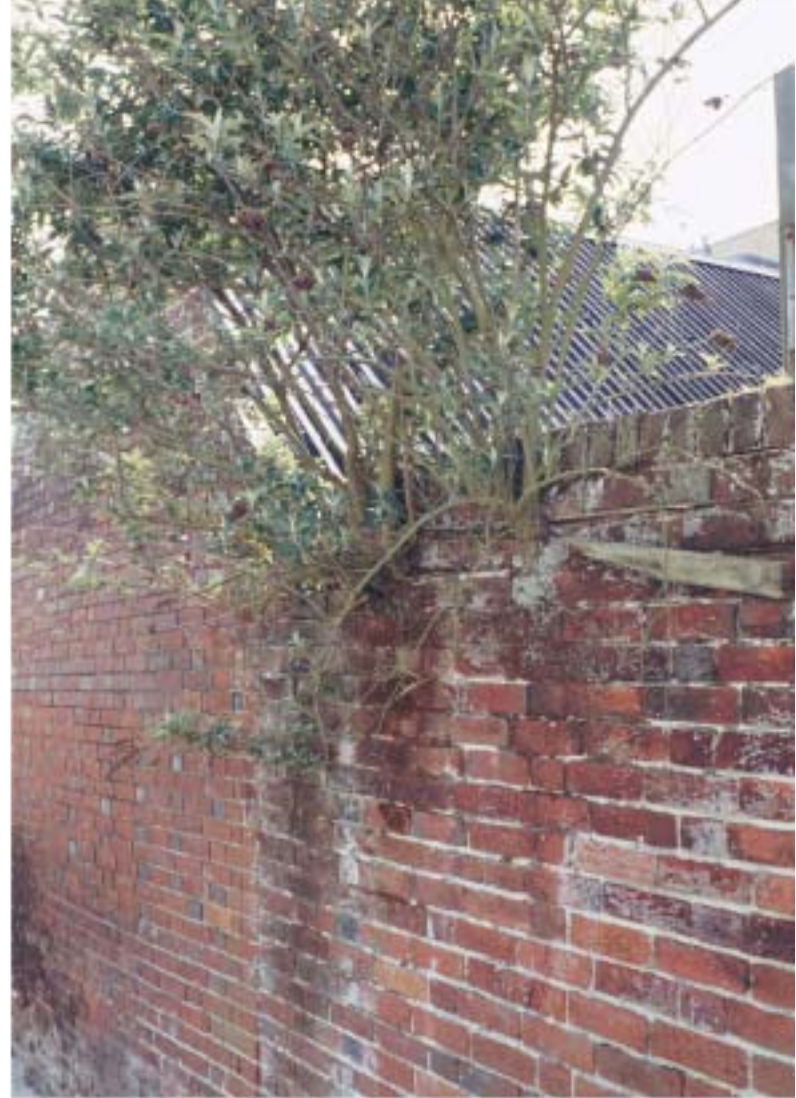
Vegetation growth in brickwork may cause significant damage if left unchecked.
