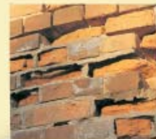
The use of a hard cement mortar for pointing will cause accelerated erosion of historic brickwork.
