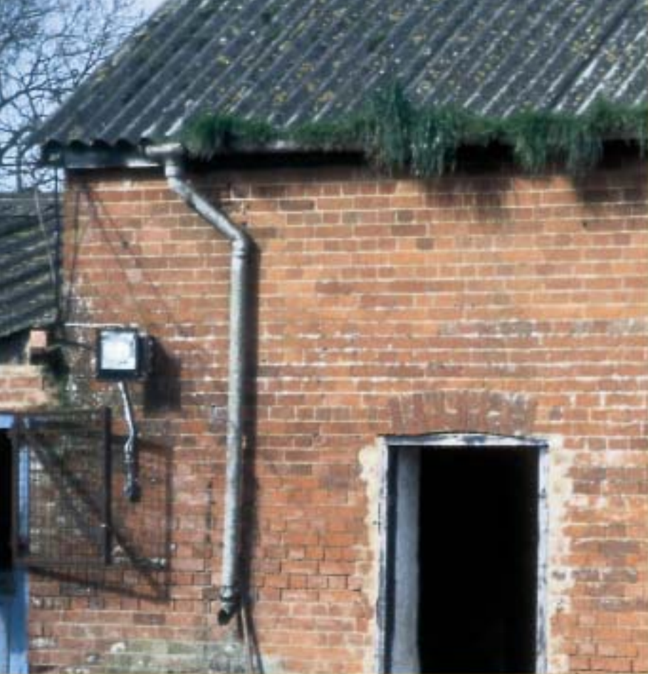
Vegetation growth in guttering
